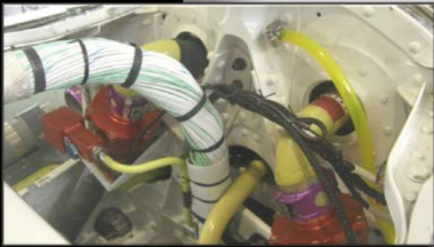
Electrical Wire Harnesses Installations
